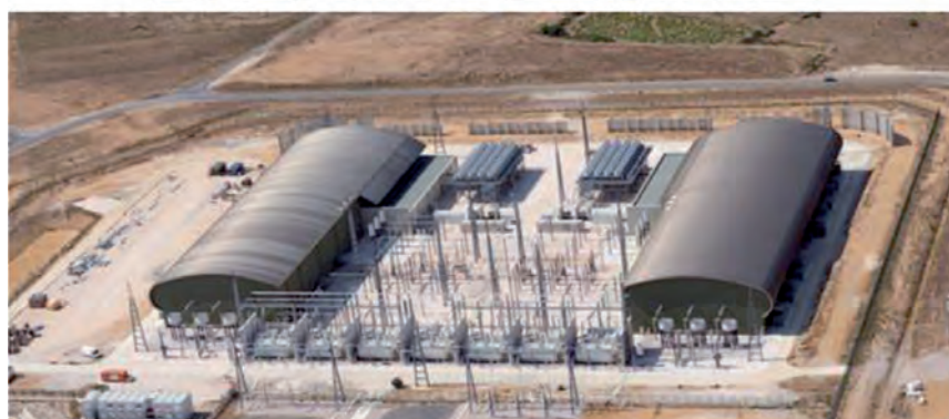
Overview of the converter stations of the 2 times 1000 MW Spain to France (INELEF) VSC dc project (CIGRE 2016)
